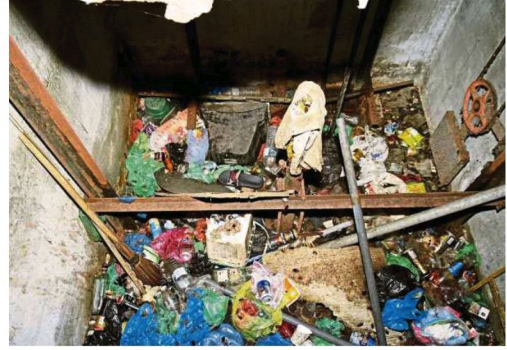
Rubbish thrown inside a broken lift shaft at the apartment block.
