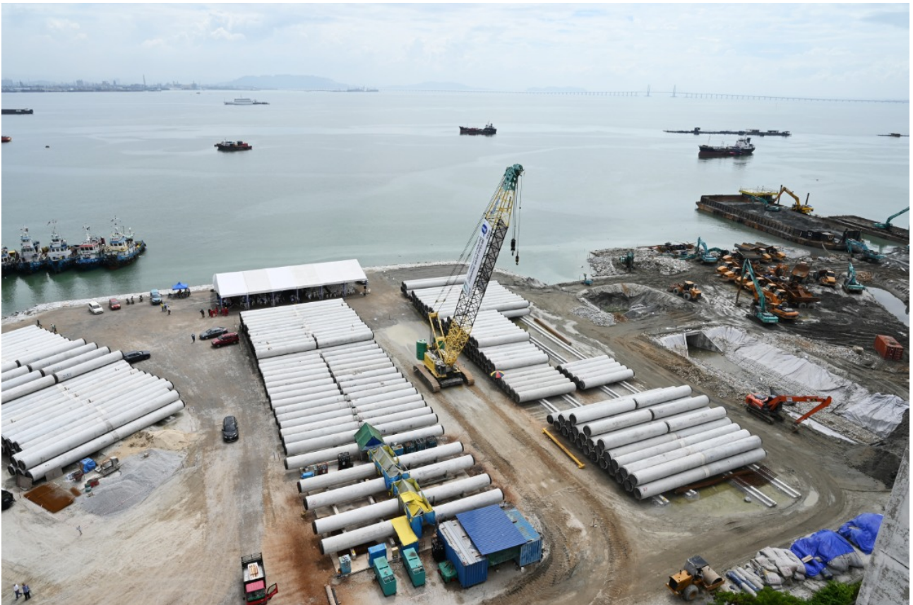
An aerial view of the rows of mild steel pipes at Macallum that would be laid across the channel for the 3rd Penang Submarine Pipeline project from George Town to Butterworth.
