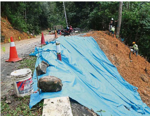
Tarp protecting a slope on the road leading to Air Itam Dam.
