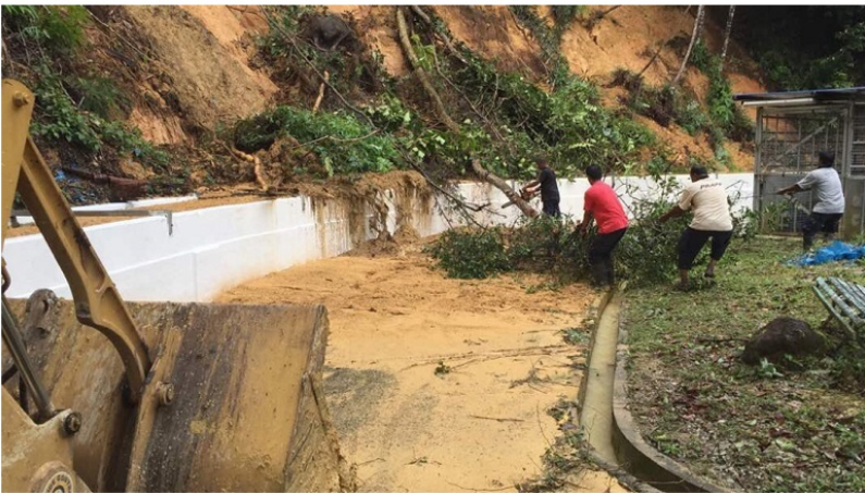
PBAPP personnel clearing fallen trees and debris at the aqueduct in the Guillemard water treatment plant in Penang. — Picture courtesy of PBAPP
