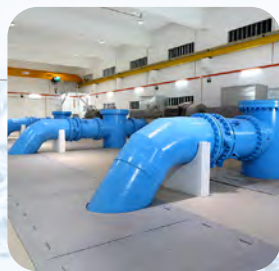
● Treated Water Pumps
